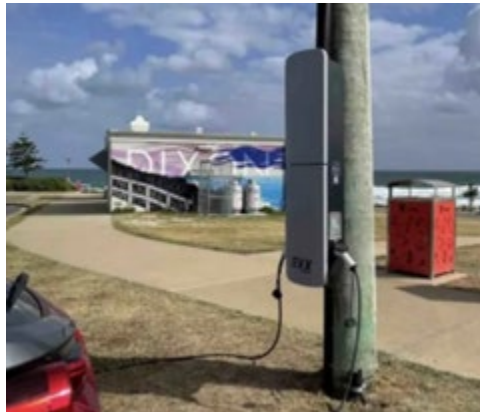
Figure 7. Utility-mounted curbside charger in Newcastle, Australia. Source: Ausgrid
