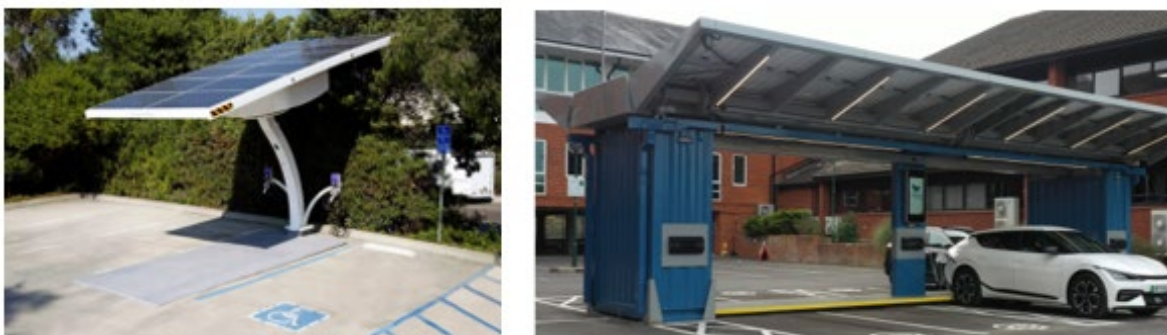
Figure 6. Mobile and containerized charging solutions: Beam Arc (left) and Papilio3 in the UK (right). Source: Beam, 3ti.
